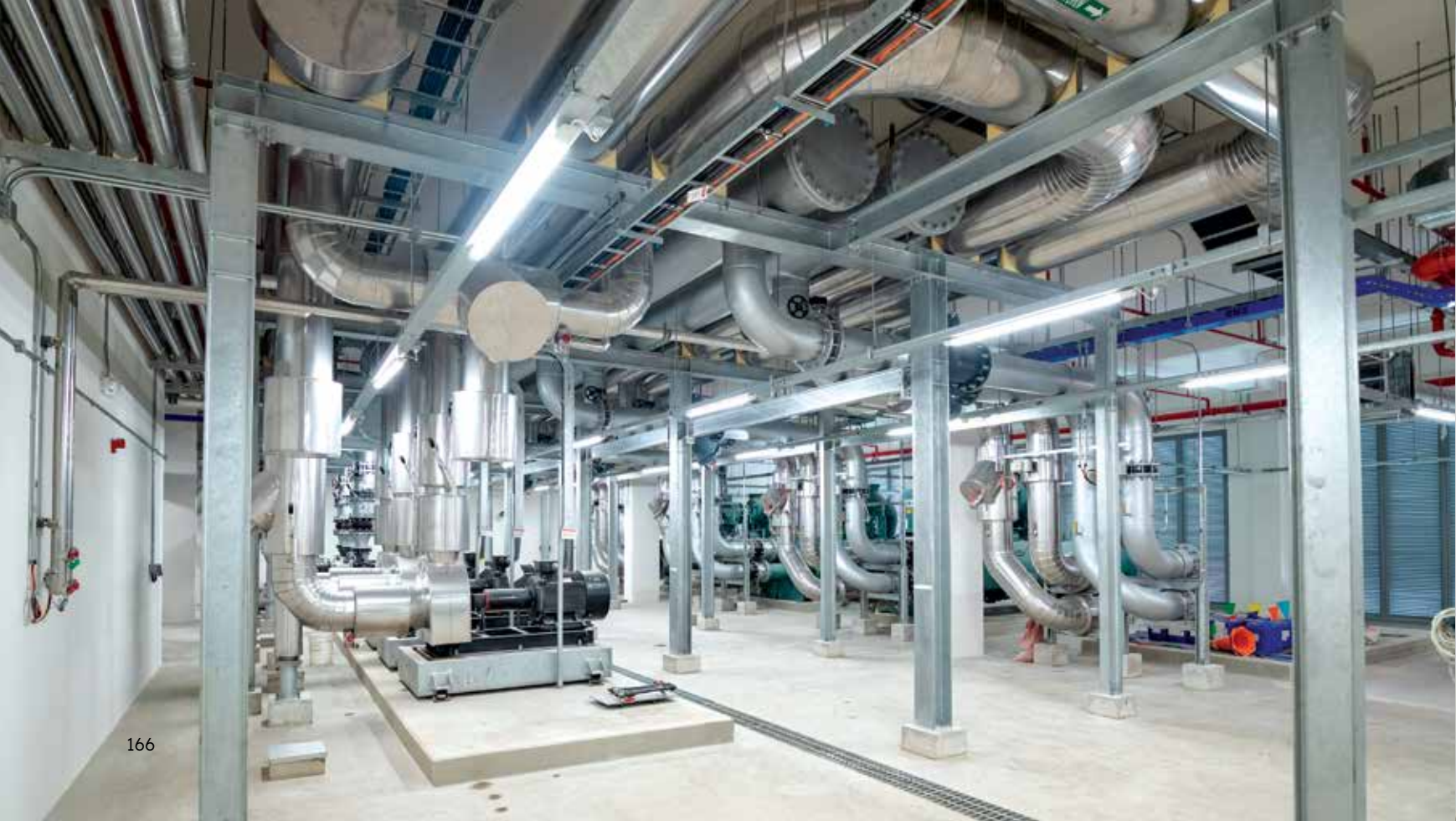
BIM-coordinated Chiller system featuring optimized layout, precision-machined support racks, and high-quality MEP installation at the Pandora Production Vietnam plant project (HCMC).
